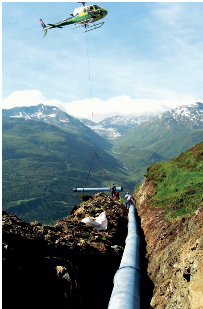
A turbine pipeline
